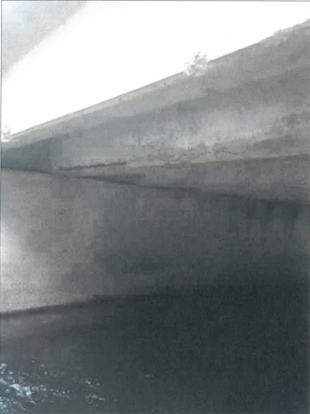
Photo 3. Damaged bridge girder and exposed rebar.
