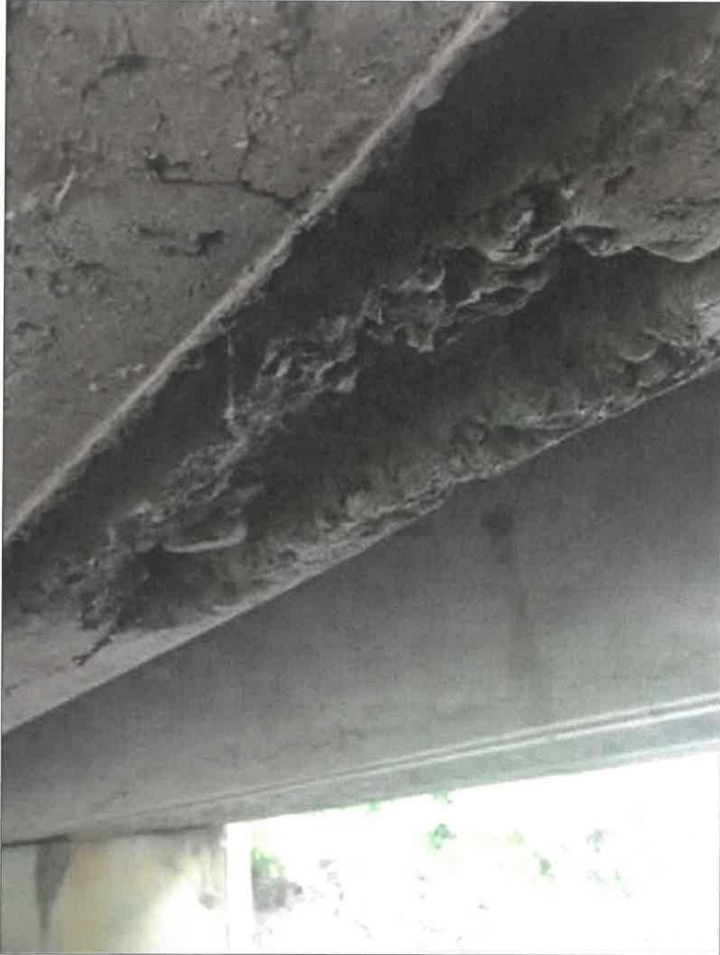
Photo 4. Damaged bridge girder and exposed rebar.
