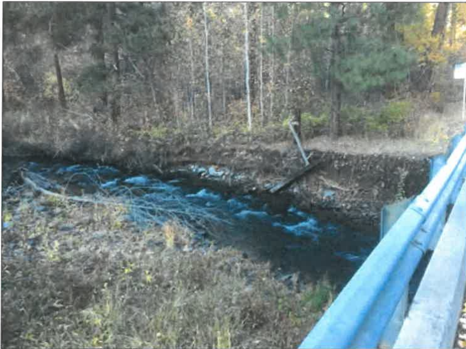
Photo 5. Scour on the north bank of Manastash Creek.
