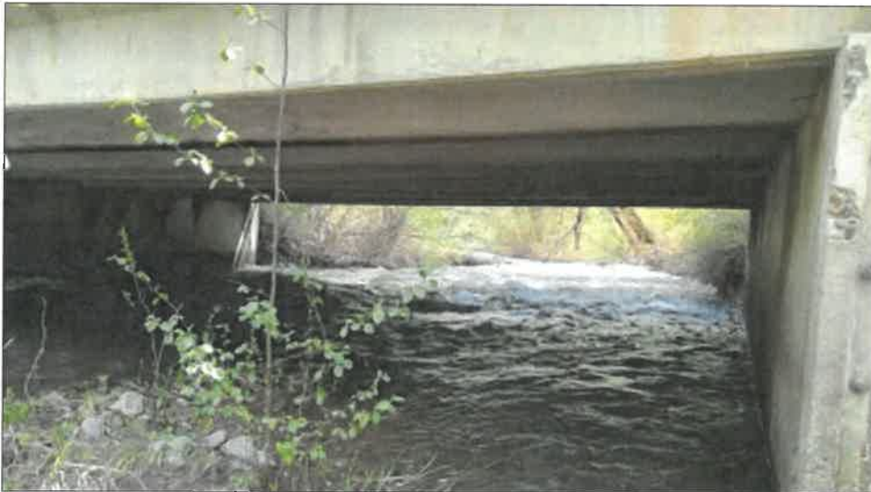
Photo 2. Damaged bridge girder.
